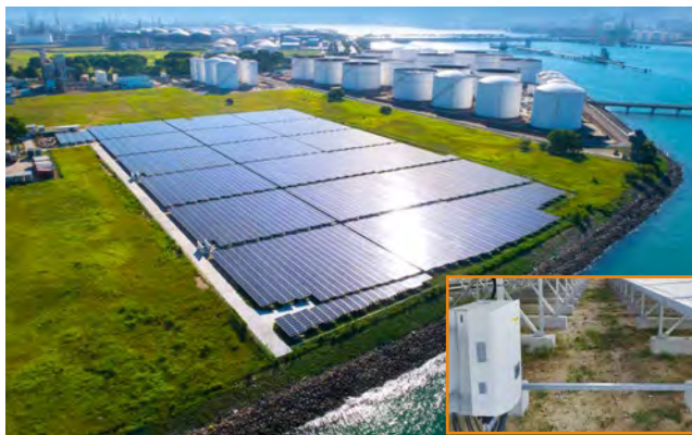
JTC Solar Farm, Singapore 5MW
