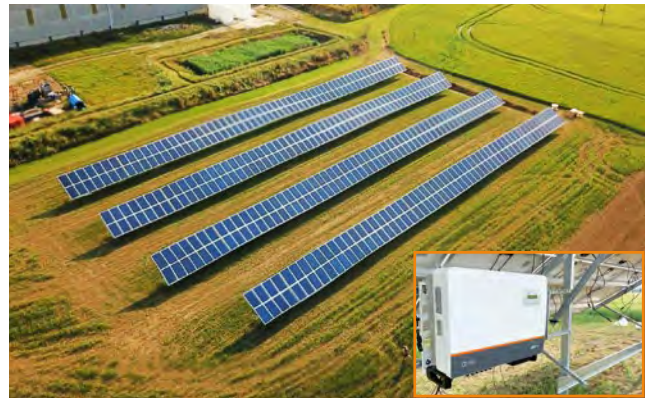
Lincolnshire, UK 140kW
