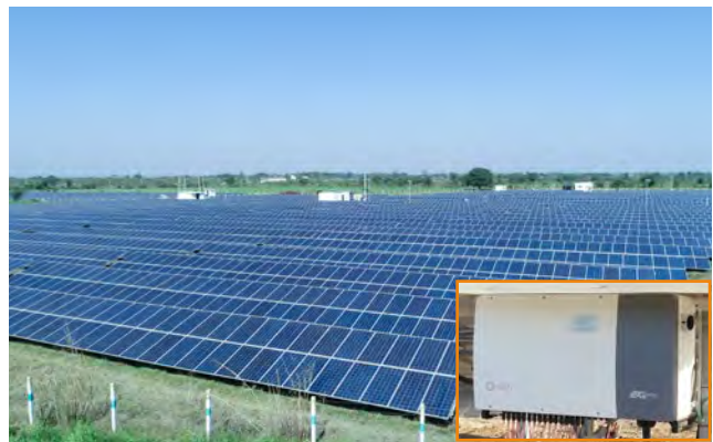
Soleos Energy Project, India 2MW
