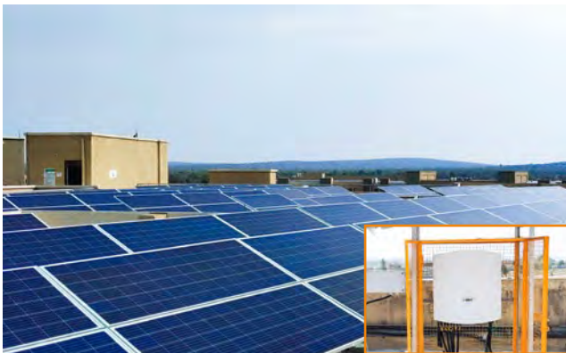
Police Training Project, India 450kW
