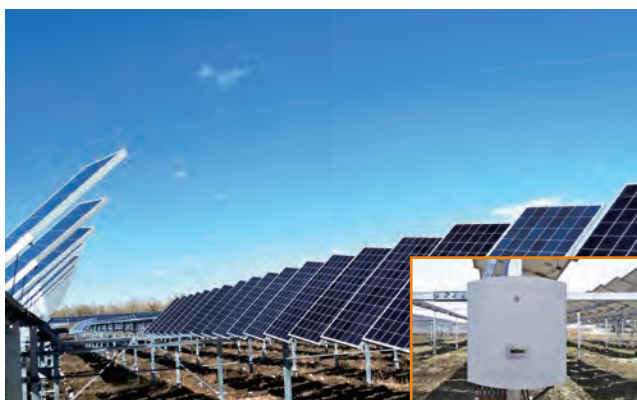
Hebei Zhangbei Agricultural-photovoltaic hybrid PV plant 50MW
