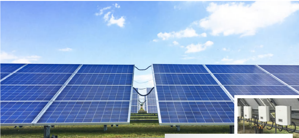
Mexico 20MW Solis-20K-HV
