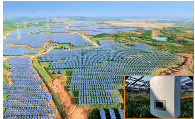
Zhejiang Hangbu Agricultural-photovoltaic hybrid PV plant 30MW
