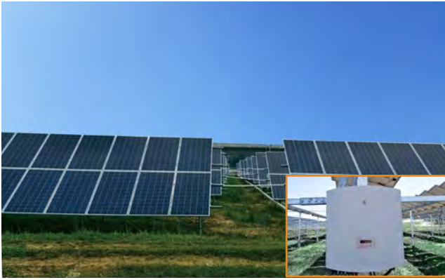
Hebei Zhangjiakou poverty alleviation PV Plant 5.1MW
