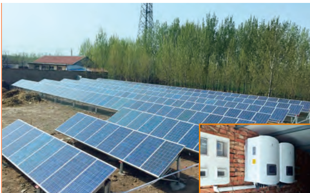
Shandong Leling poverty alleviation PV Plant 50kW
