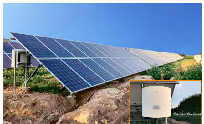
Hebei Qinghuangdao poverty alleviation PV Plant 5MW
