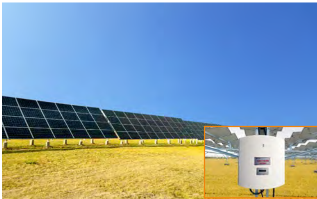
Huaneng Yimin surface mine PV plant 20MW
