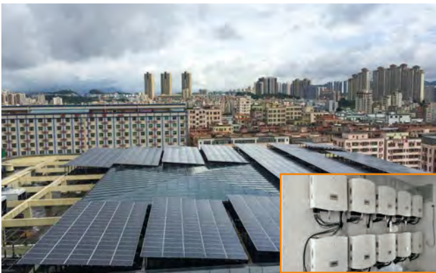
Shenzhen Jiangnan Times Building 600kW
