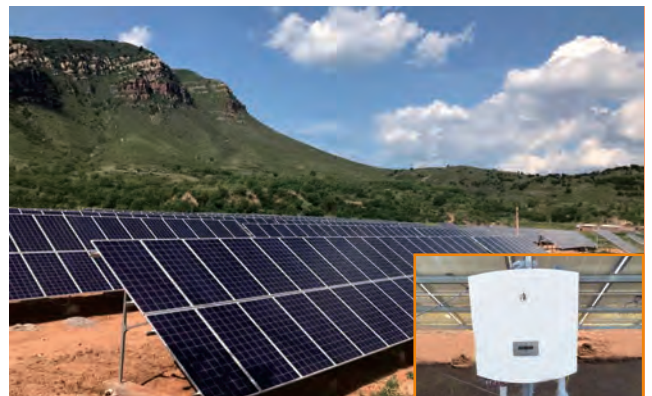
Shanxi Xiyang poverty alleviation PV Plant 7.2MW
