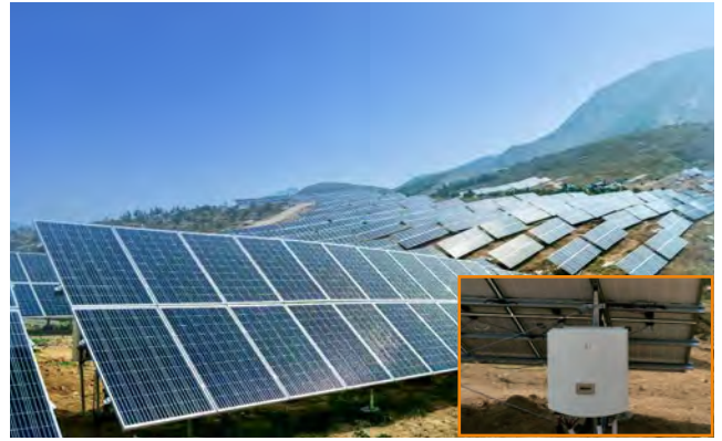
Liaoning Yingkou Jiuzhai PV plant 20MW
