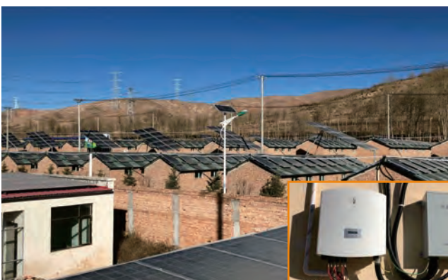
Qinghai HuzhuBanyan poverty alleviation PV Plant 2MW
