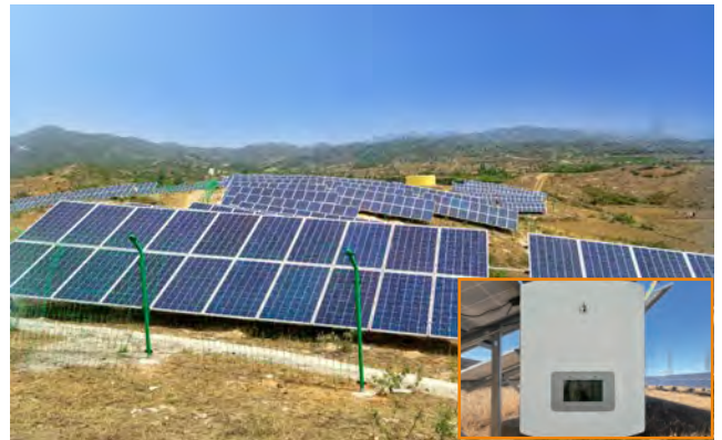
Hebei Qinghuangdao poverty alleviation PV Plant 9.7MW
