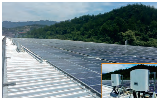
Hainan JiuLongGlass 1.7MW
