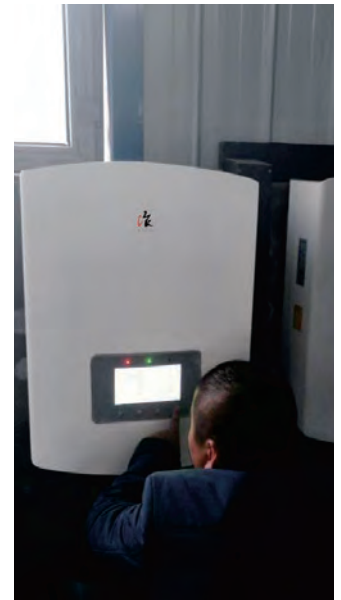
Heilongjiang PV plant
