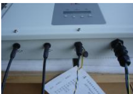
Picture 1. Ginlong Inverter
