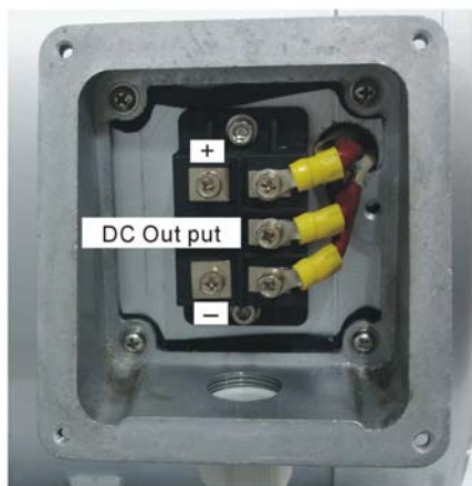
GL-PMG-5K electrical box
